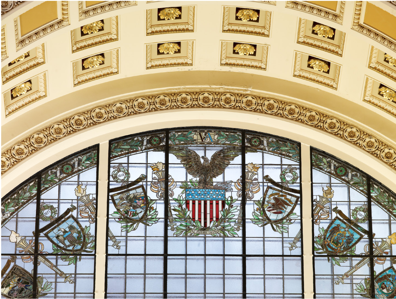
MAIN READING ROOM. DETAIL OF STAINED GLASS WINDOW AND COFFERED ARCH INSIDE ALCOVE. LIBRARY OF CONGRESS THOMAS JEFFERSON BUILDING, WASHINGTON, D.C. CAROL M. HIGHSMITH 2007
